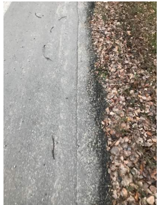
Existing Micro-Surfacing on Sunset Drive
