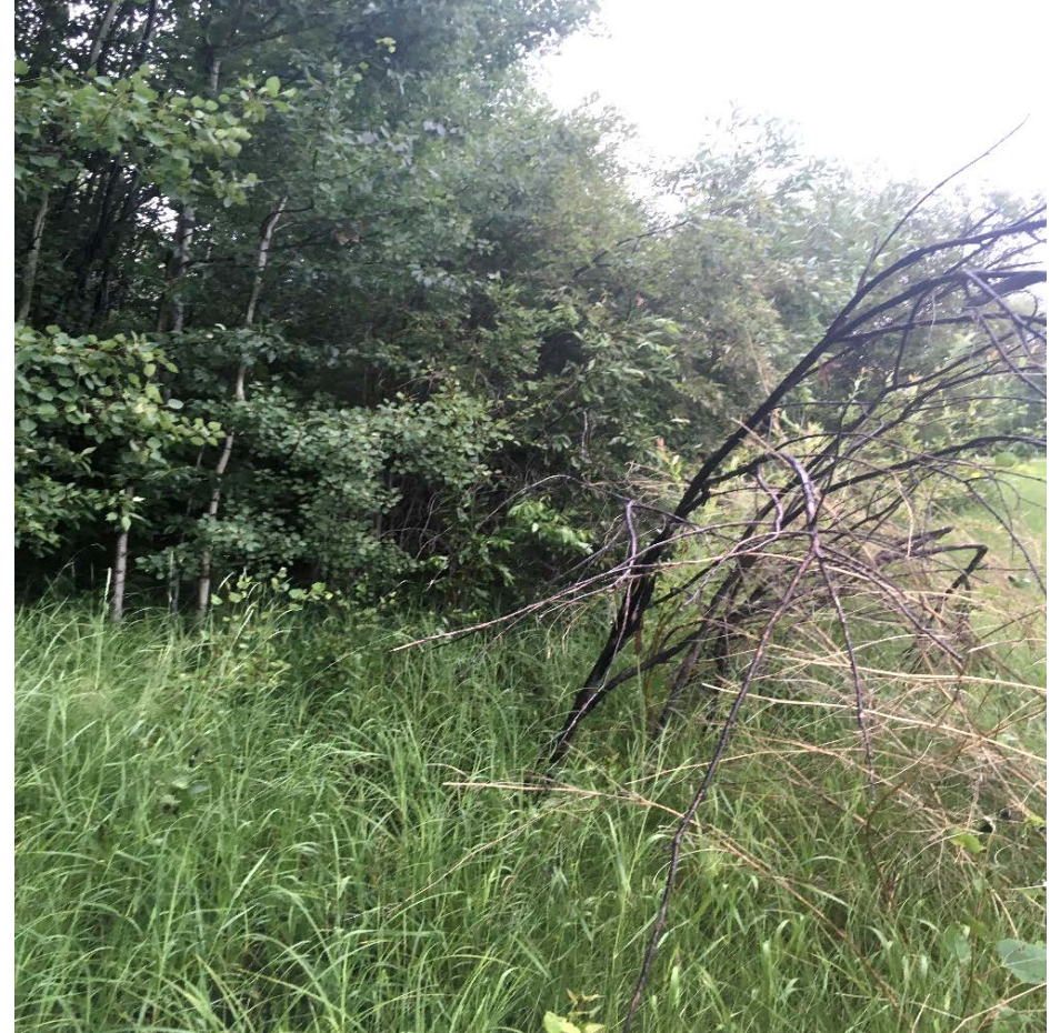
Photo 30 – Culvert I04 outlet, blocked by shrubs, facing east.
