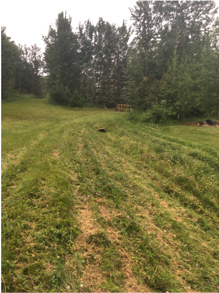
Photo 7 – Railway embankment from behind Lot 53 (48 Street), culvert D08 inlet (center), facing south.
