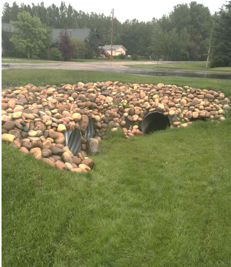
Photo 15 – F03 and F04 culvert inlet (left) and F05/F06 culvert outlet (right), facing east.
